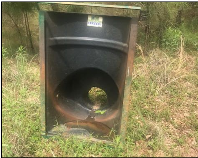
Steel water control box resolves dam issues
